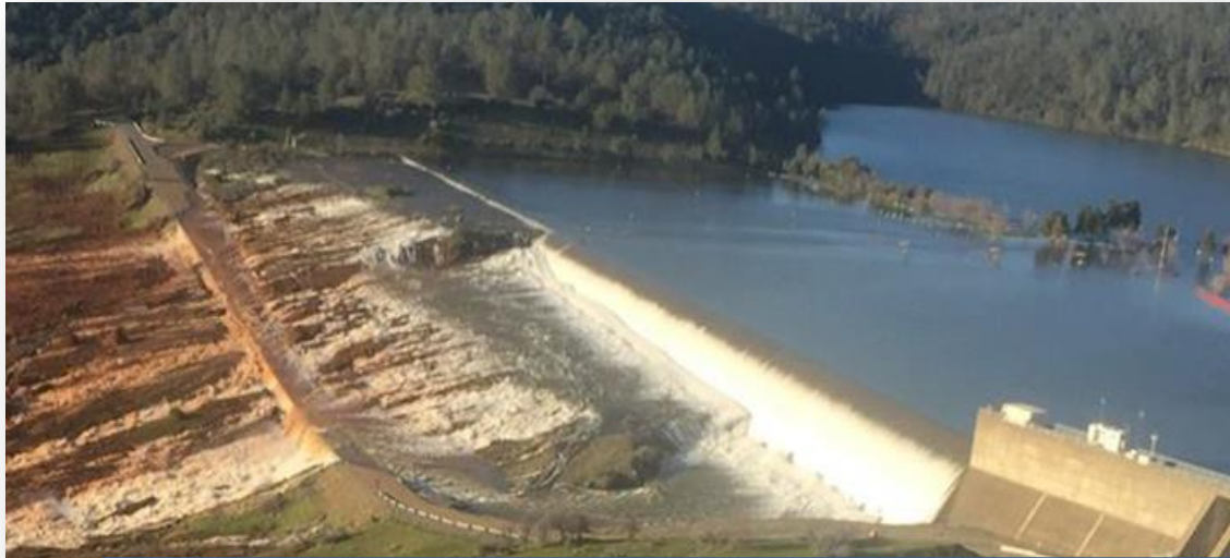
Oroville Dam, spillway damage, 2017
