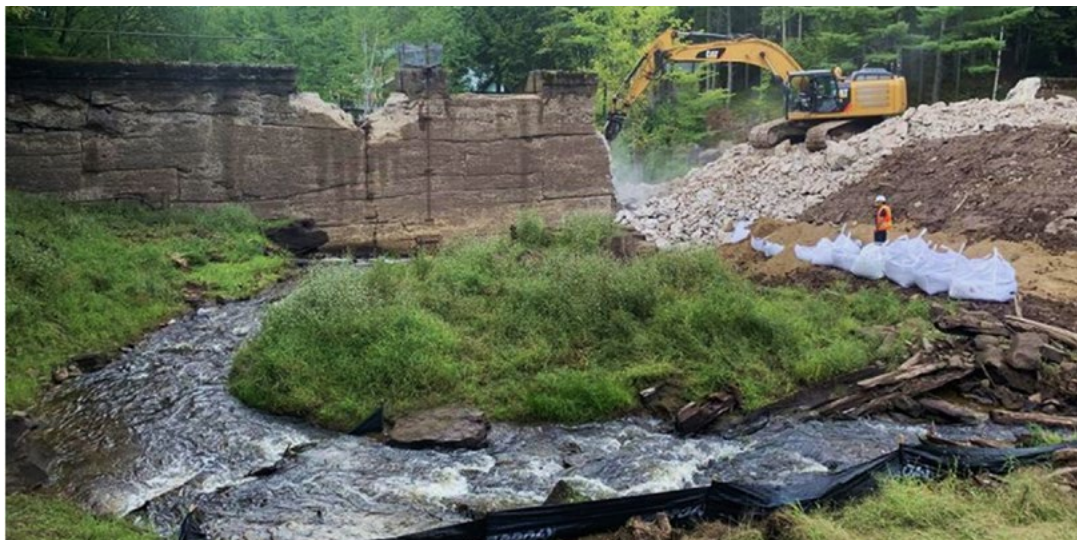
Demolition of the Campbell Creek Dam. (Photo: Nathan Wilbur/Atlantic Salmon Federation with permission)
